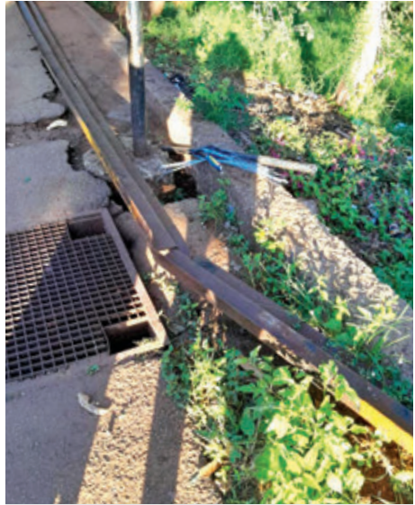
The costly damages caused by cable theft.
